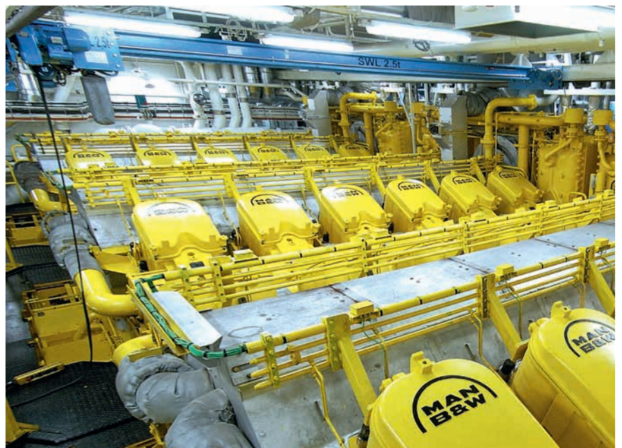
Engine Room Crane SWL 2.5t Class LR
