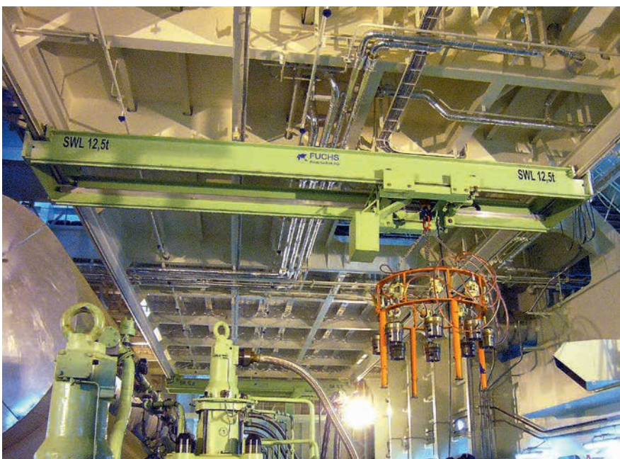
Engine Room Crane SWL 12.5t Class LR
